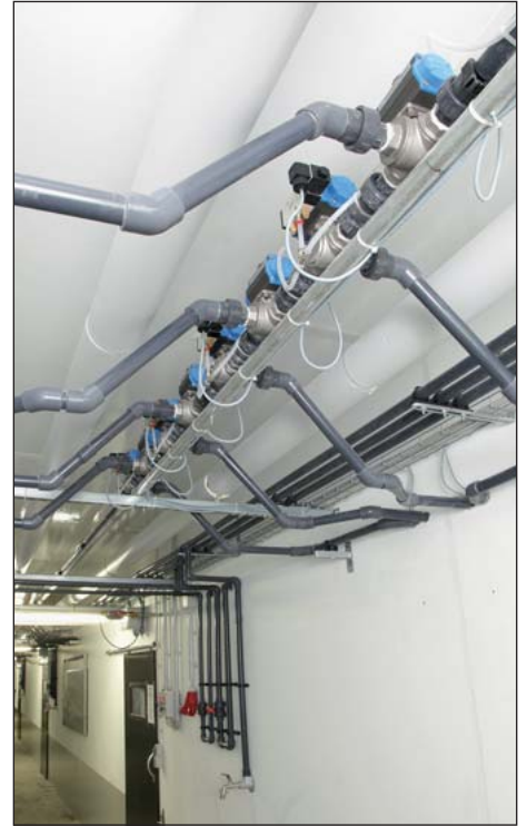
Feed valves installed in the central corridor
